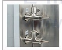
SS Water tap & Gas tap
